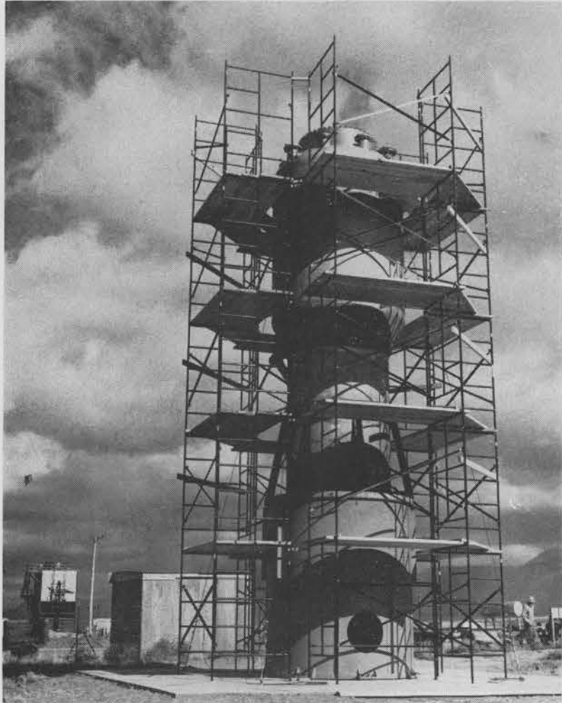
REACTOR PRESSURE VESSEL stands in Area III undergoing inspection prior to installation. Sandia's Engineering Reactor Facility is currently under construction and scheduled for completion early in 1961. Cost of construction is placed at $1,808,600.
