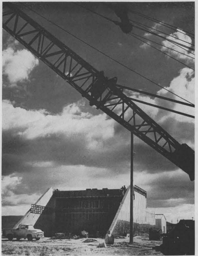
RADIANT HEAT FACILITY in Area III takes shape as workmen work on the inner walls of the environmental test facility. Construction will cost $279,990 and will be completed in January.
