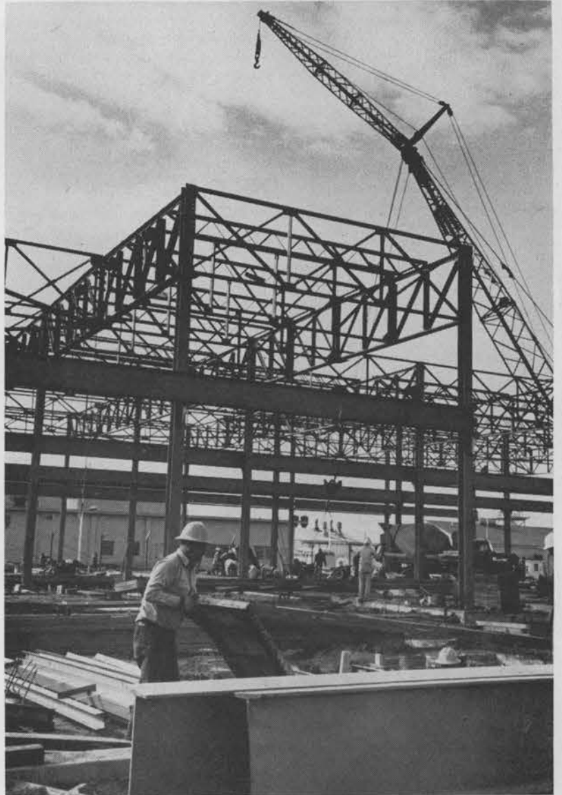
NEW SPECIALTIES BUILDING for the Development Shops (Bldg. 841) is under construction in Area I. Steel framework of the new building is shown in this photograph. Valued at $977,700, construction project is scheduled for completion about June 1960.
