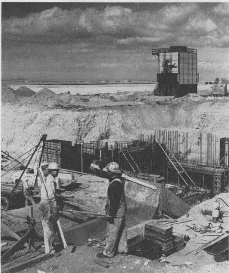
HUGE HOLE in the earth marks location of Sandia Engineering Reactor Facility in Area III. Workmen are currently pouring concrete base for the reactor pressure vessel. In the background can be seen the partially constructed cooling tower.
