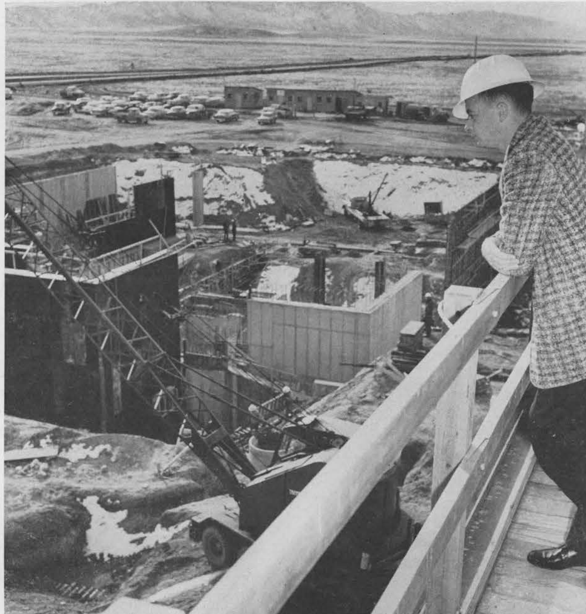
CONSTRUCTION PROGRESS at the Sandia Engineering Reactor site in Area III is viewed by R. M. Jefferson (1626), foreground, from the top of the recently completed three-story reactor cooling tower. Photograph shows thick steel and concrete going up. Operation is expected in 1961.
