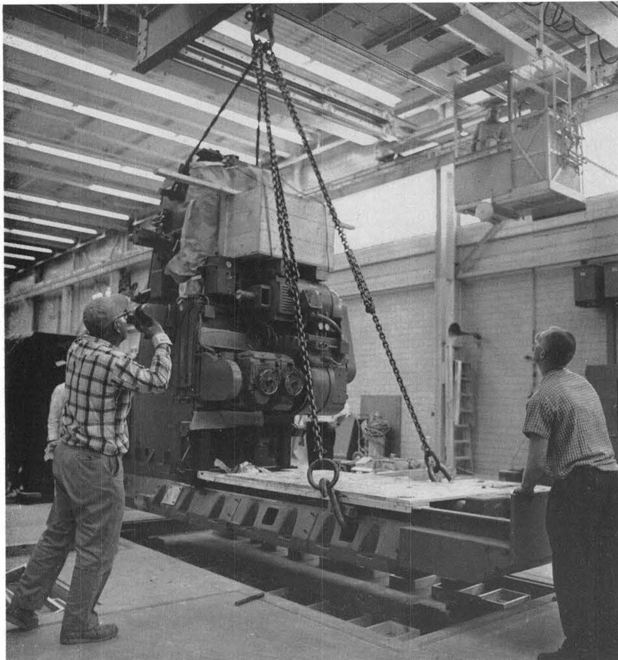
EASY DOES IT. Several weeks ago, installation of Omnimil OM3, numerically-controlled milling machine, started in Bldg. 840. Two overhead cranes were used to
