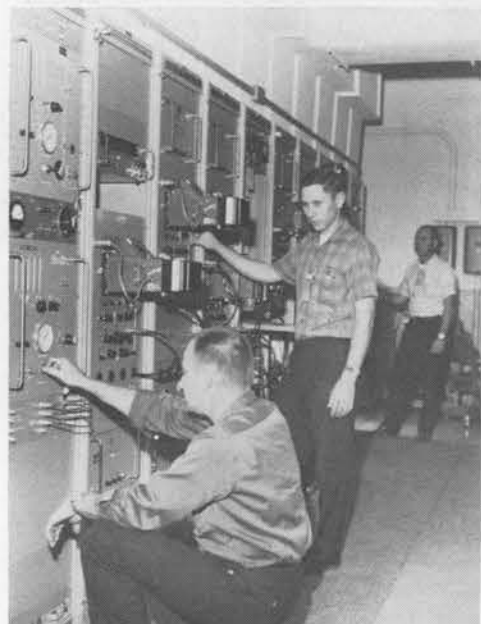
CONTROLS FOR ONE FIRING CHAMBER are set just before a test by (l to r) photographer Gordon Bennett, technician Steve Folkendt, and test engineer Gene Anderson. Gene holds the master key for the panel, which closes an interlock to prevent accidental or inadvertent actuation of the equipment.
