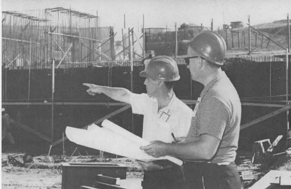
PART OF AREA 8 CONSTRUCTION is reviewed by Dick Myers (left) and Joe Sladky. The building going up in the background is the new HE environmental test laboratory, Building 976.
