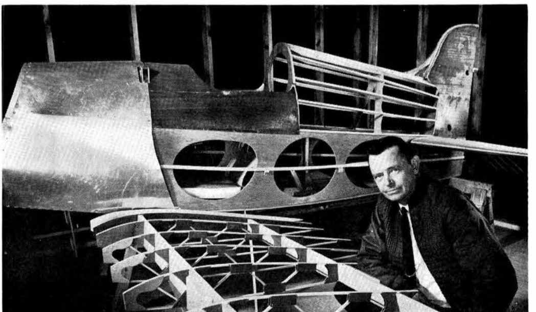
CONSTRUCTION DETAILS of Lew's airplane are revealed in this photo taken about a year ago. He used fir plywood and fir stringers for most of the construction. Sheet metal is aluminum.
