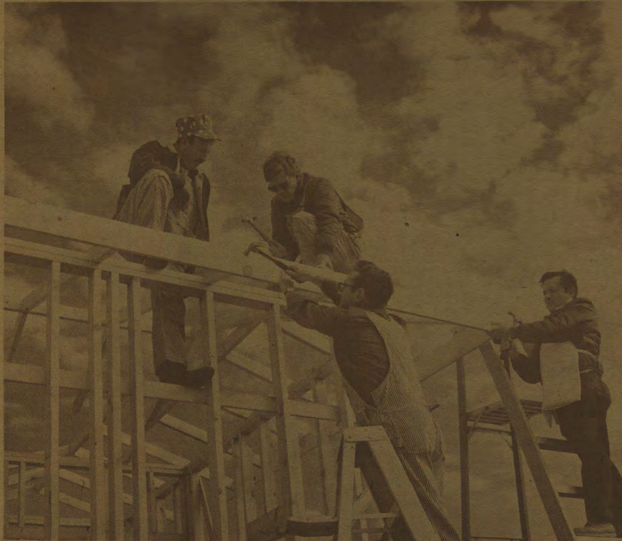
SEVERAL kinds of framing construction are represented in this storage shed being built by apprentice carpenters. Instructor Frank Lesperance, left, gives the word to Jerry Smith, Al Ayott and Milton George (all 7513). The Plant Technician apprenticeship program requires 10,000 hours of classroom and field training.
