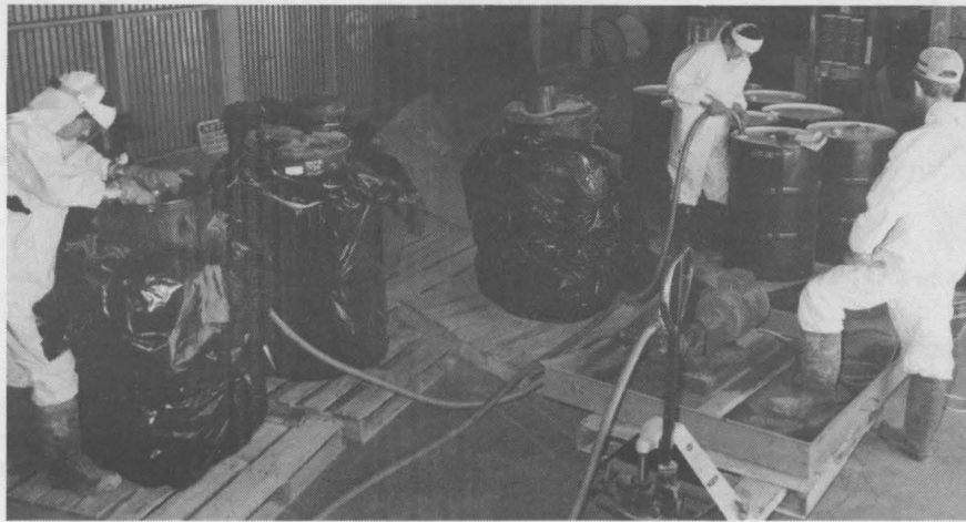
CONTRACTORS REMOVE PCB fluid from old utility transformers before they are shipped to an approved landfill for disposal. Sandia is currently substituting non-PCB insulating oil in all transformers in use at the Labs.
