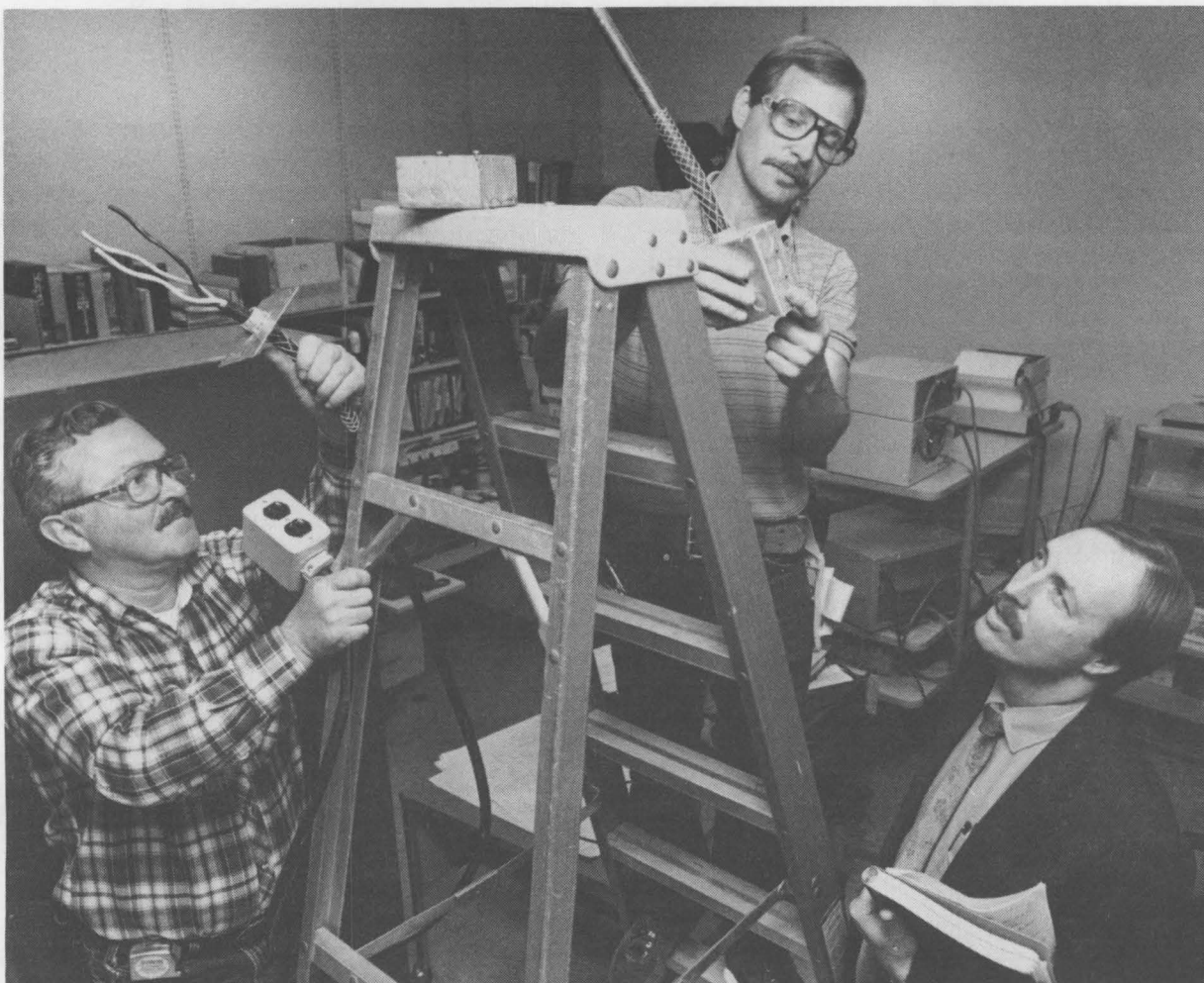
TAKING CARE of one of 35,000 findings — most minor — listed by inspection teams during phase one of Sandia's ES&H Compliance Initiative, Ron Young (7813, left) and Doug Wilfon (7813, center) replace a metal electrical-outlet box with a new nonmetallic one and make other electrical repairs. Jim Smith (7823, right) coordinates ES&H compliance activities for Facilities 7800.
