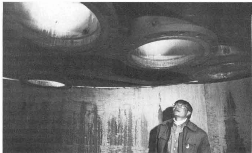
BENEATH THE TANK that forms the outer vessel of CYBL, T.Y. Chu (6422) examines access ports for diagnostic instruments and other hardware.
