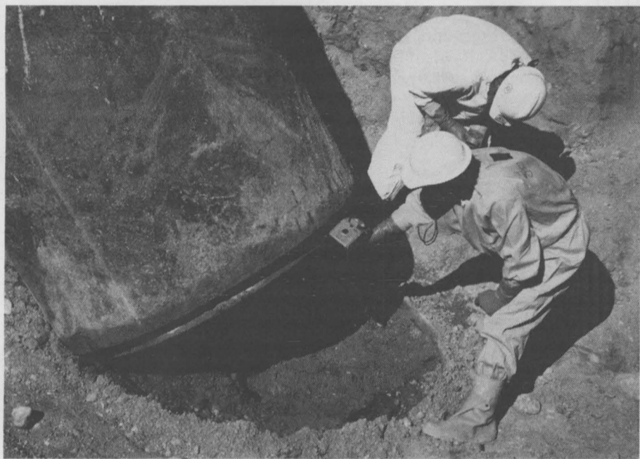
URANIUM PIT CLEANUP — Workers examine soil beneath a tank being removed from an environmental restoration project site in Sandia's Tech Area 2. Remediation of the site involved removing material from four uranium calibration pits DOE had used between 1978 and 1984 to test and calibrate uranium exploration tools.
