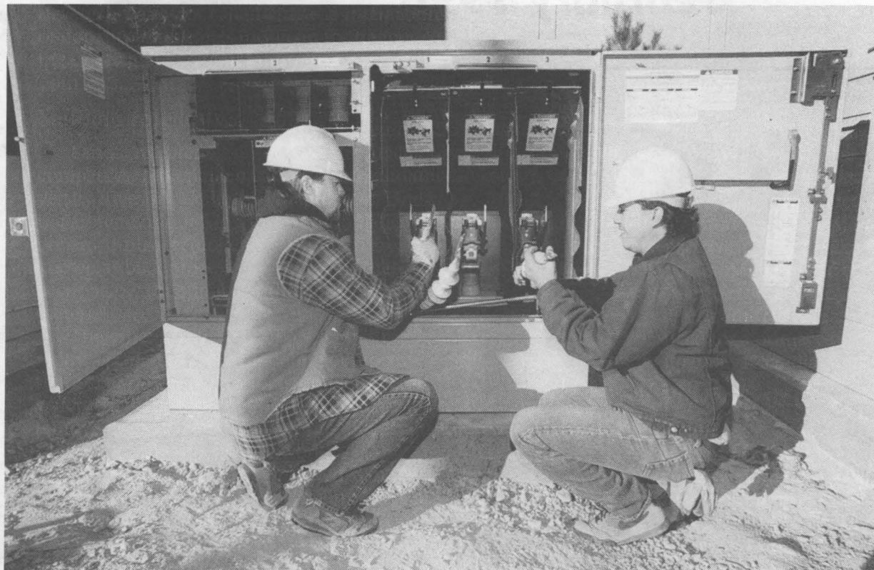
REWIRING THE LABS — J & S Electric employees Leonard Gragg (left) and Ben Cordova work on terminating high-voltage cable. Their work is part of Sandia's $37 million Power Systems Modernization project.
